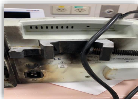
(Figure 2): Damaged Infusion Pump due to unapproved extension cord.
