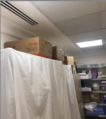
Boxes were found reaching the ceiling
