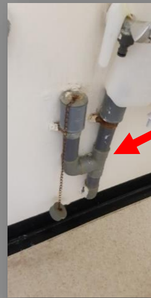
Water drainage for Dialysis rusty all rooms
